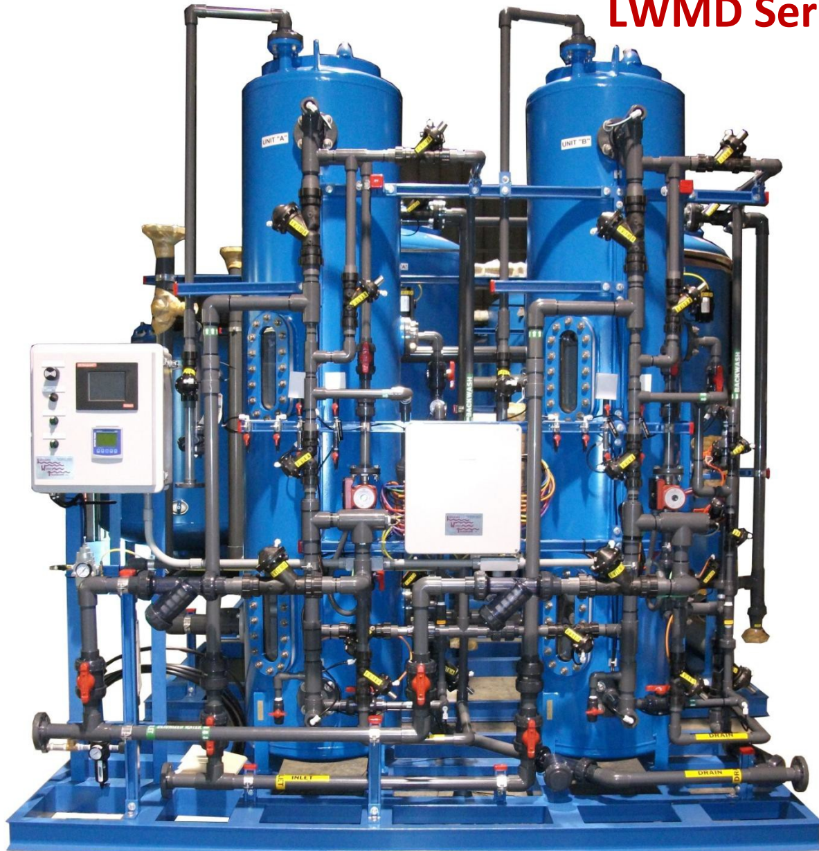
Industrial Mixed-Bed Polishing System
